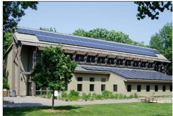
Roof-mounted photovoltaic solar power system
