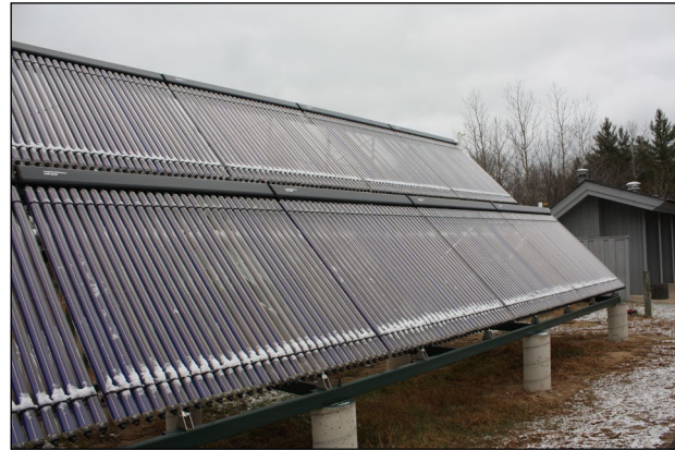
Ground-mounted indirect solar hot water system
