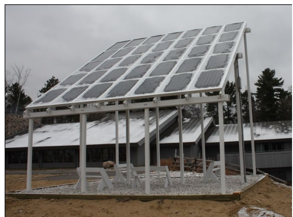
Double-sided, ground-mounted photovoltaic solar power system
