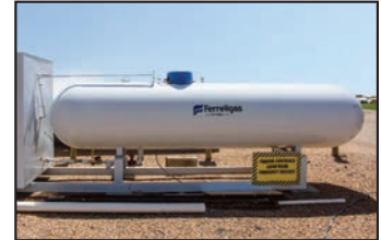
ASME Above-ground LP Tank
