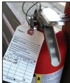
Fire extinguishers should be inspected periodically.
