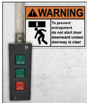
Warning sign accompanies three-button control switch.
