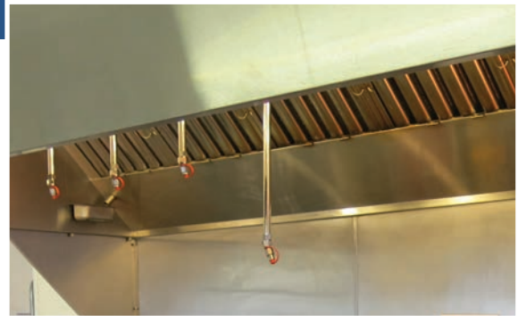
The nozzles above the cooking equipment spray wet chemicals once any smoke or grease-laden vapor is detected.
