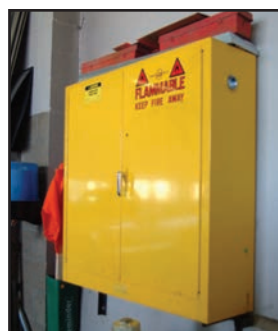
Flammable materials storage cabinet
