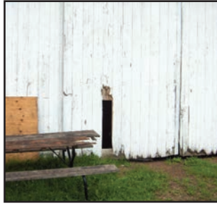
Unchecked buildings could lead to greater property damage and safety hazards.
