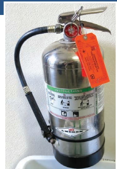
Keep a class K fire extinguisher within 30 feet of deep fat fryers.
