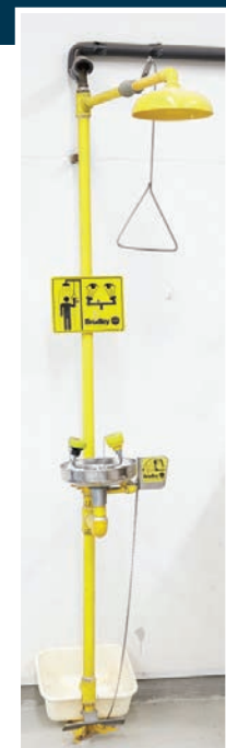
Emergency eyewash and shower stations allow employees or volunteers to rinse off in case of chemical contact.
