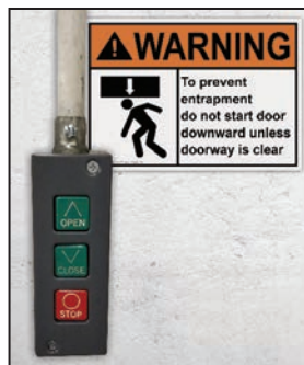
Warning sign accompanies three-button control switch.
