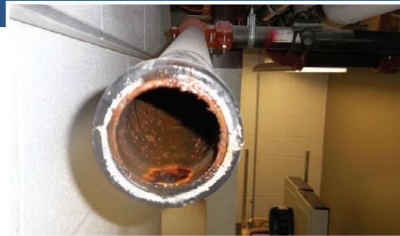
Corroded pipes may not activate a fire suppression system when needed, or activate it unexpectedly.
