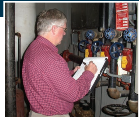
Keep sprinkler systems operational with routine inspections, testing and maintenance.
