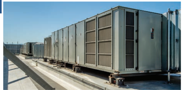
Routine tests and inspections keep HVAC systems running smoothly.
