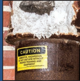
Friable pipe insulation
