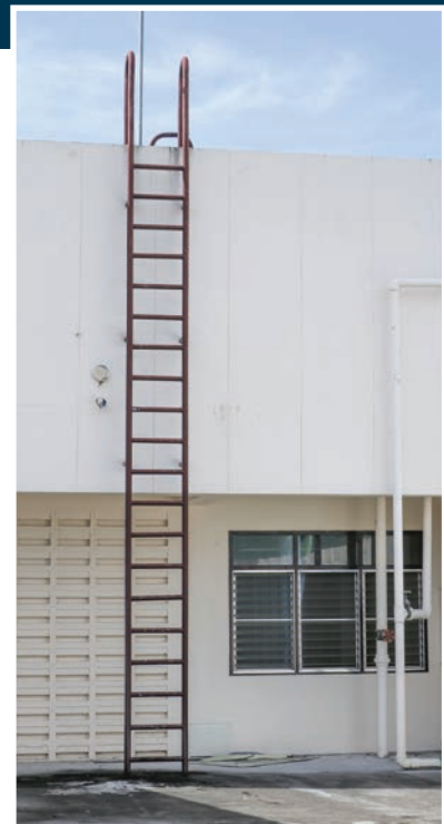
Existing fixed ladders should be updated to include personal fall protection or ladder safety systems.
