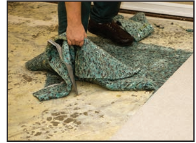
Fix leaks in roofs, walls and plumbing so mold does not have moisture to grow.
