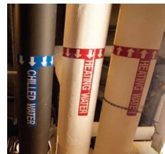
Clearly labeling pipe contents can help identify leaking substances.
