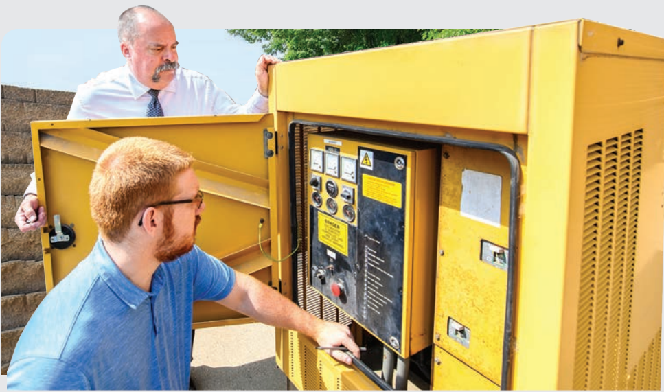
Facility Manager Kevin Coleman and facility maintenance technician Nathan Haupt conduct a routine inspection of the MCIT building's generator.
